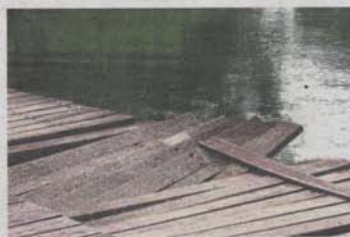
The broken wooden boardwalk in Central Park.
