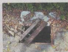
This manhole is missing its cover and poses a potential danger to park-goers.
